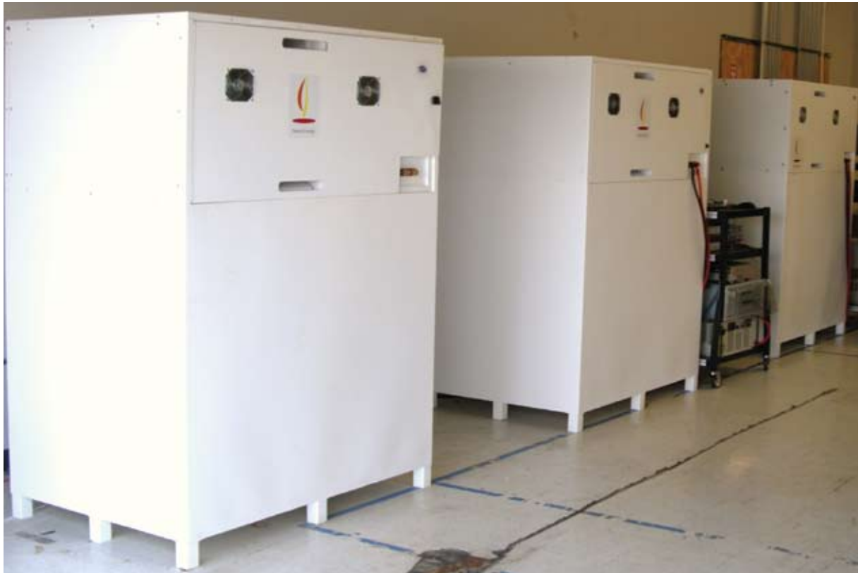
The size of large refrigerators, Deeya Energy's l-cells can provide backup power to standard cell towers for 4 hours.
